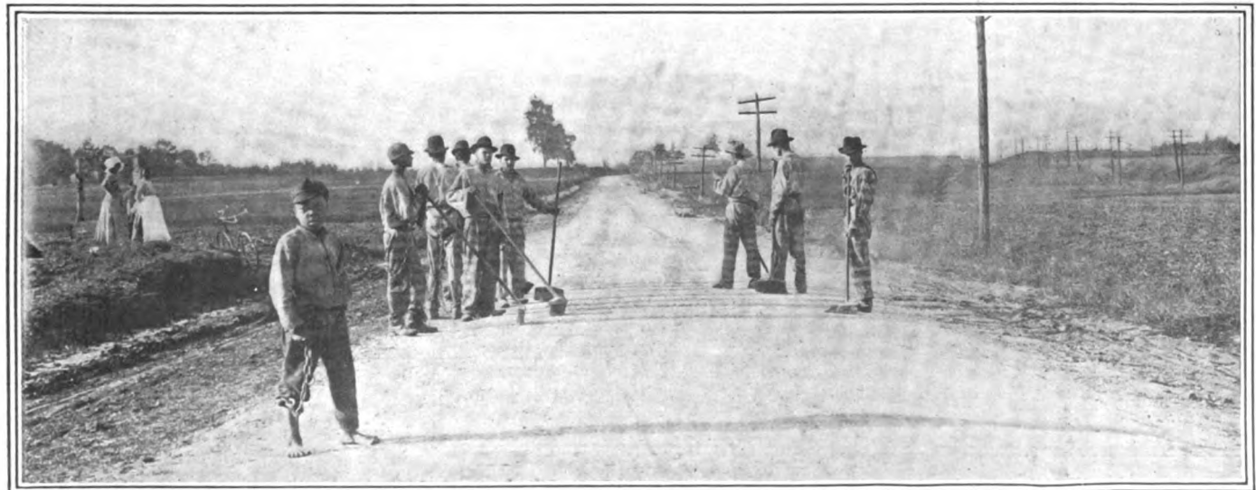
The macadam road into Concord is as good as any to be found in New Jersey
